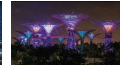
Connection of luminaires for Supertree Grove, Garden by the Bay (Singapore). Series TH400.
