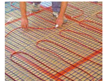
Heating cables connection.
