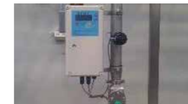
Wall mount connection on a control panel of a bottled water plant (Australia). Series TH387.
